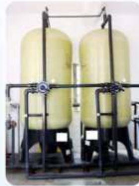
SOFTENING PLANT WITH MGF
