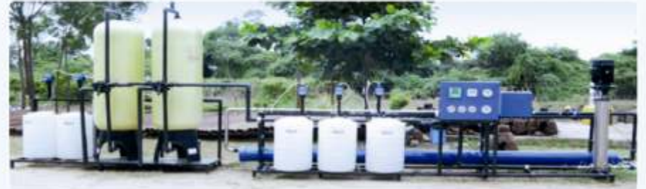
REVERSE OSMOSIS PLANT
